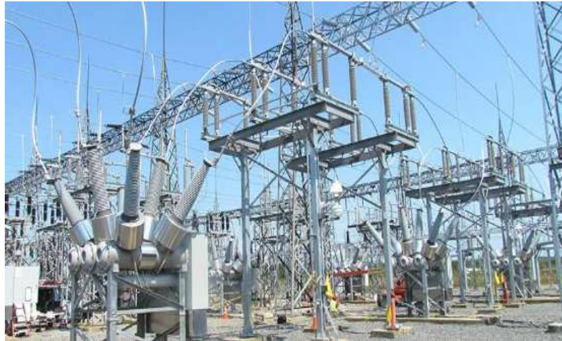
Gambar 2.2 Switch Yard (Switch Gear)
