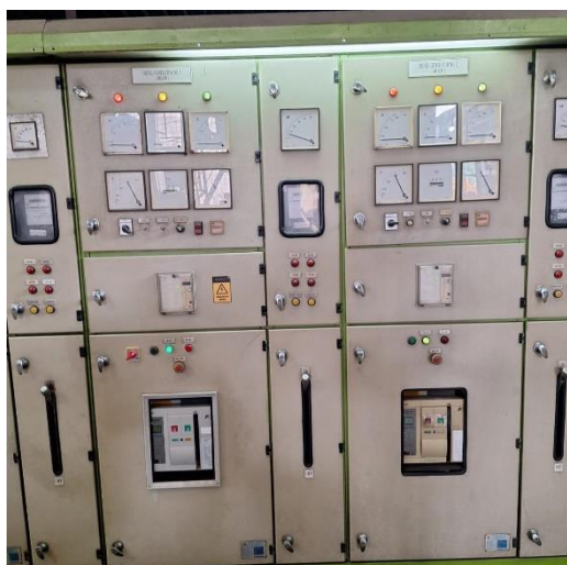
Gambar 3.6. Panel Sinkron Generator set
