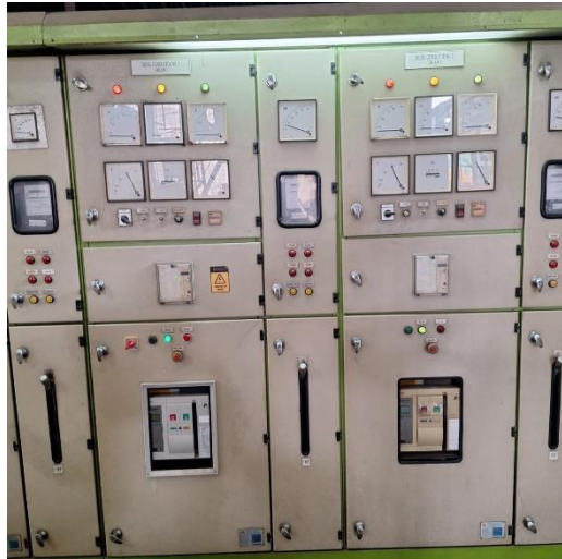
Gambar 3.5. Panel Sinkron Generator Turbine
