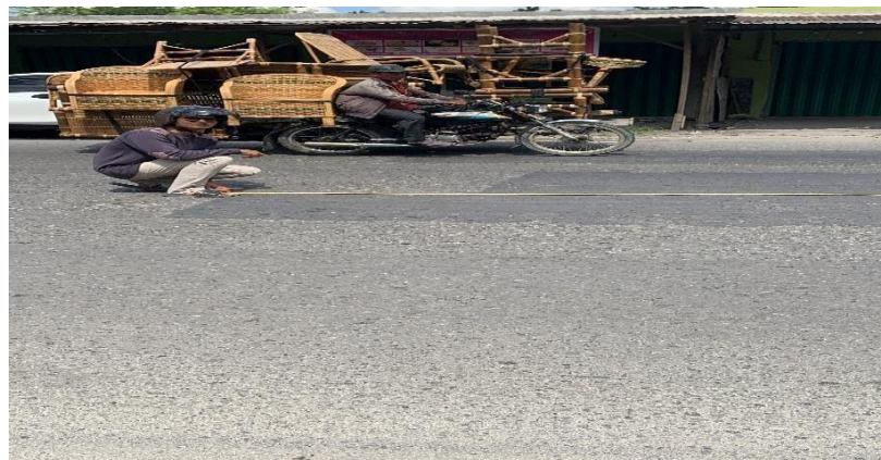
Gambar 3. 7: Tambalan ( Hasil Survey dilapangan )
