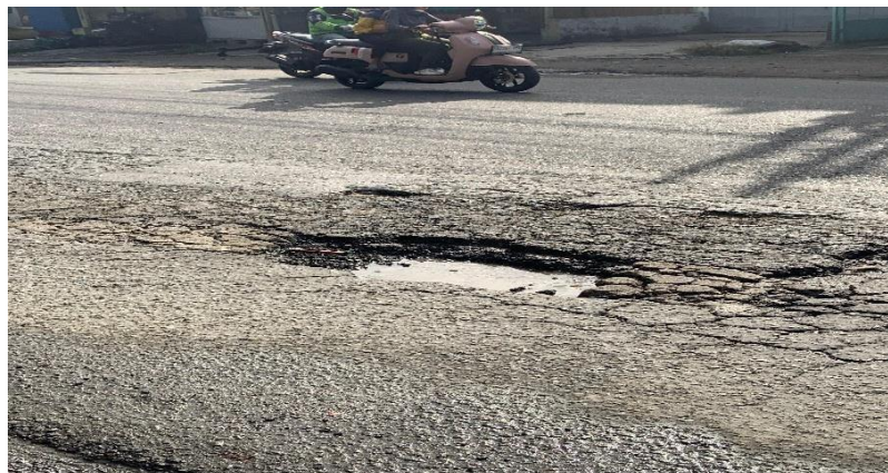
Gambar 3. 8: Lubang ( Hasil Survey dilapangan )
