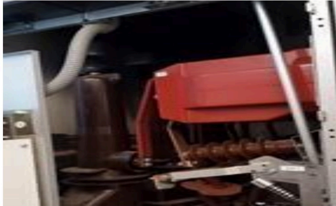
Gambar 2.15 Trafo arus ( current transformer )
